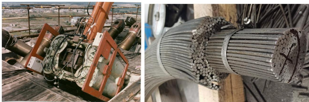
Fig. 1.8: Maintenance and inspections of prestressing system – lift-off tests and inspection of the tendon removed from the containment after 20 years of operation.
